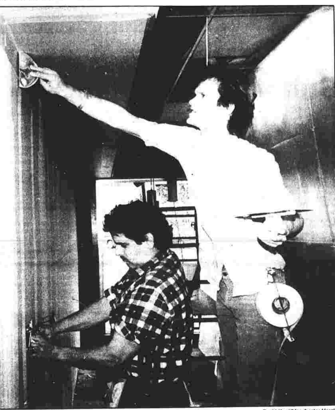
PLEASE EXCUSE ME — Greg Woodward, on stilts, works his way around Mark Tedford on a remodeling project under way at the Optical Style Bar, 763 Main St. Woodward is employed by
